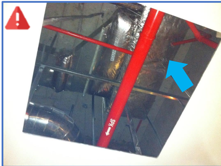
Lack of Access. Access to fan coil unit obstructed by other services despite access panel provision
