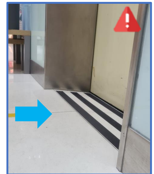
Inappropriate detailing. Floor at lift landing sloping towards lift door
