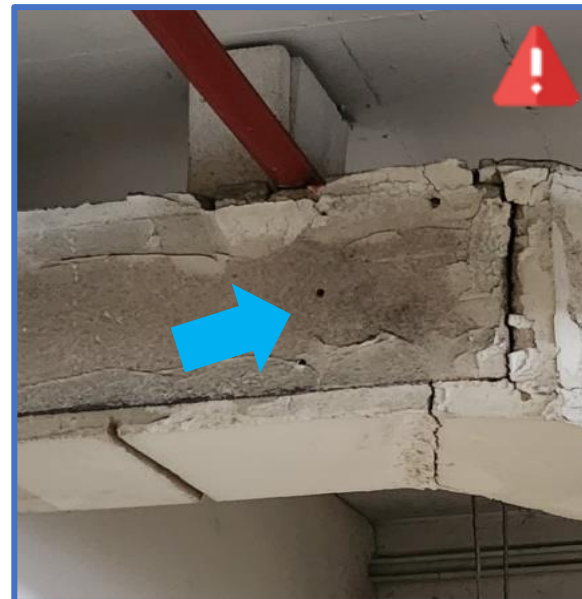
Poor Choice of material. Non-weatherproof fire-rated materials for wet riser pipe
